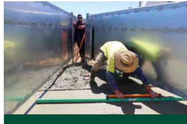
Concrete areas are boxed and screed at 100mm high as per the design specifications.
