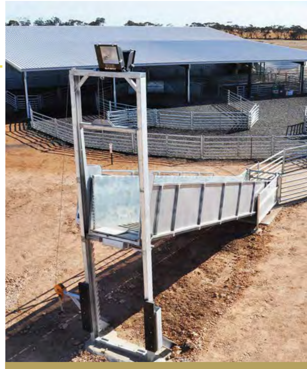
Lighting mounted on top of the ramp gantry provides a safe workplace throughout the night.
